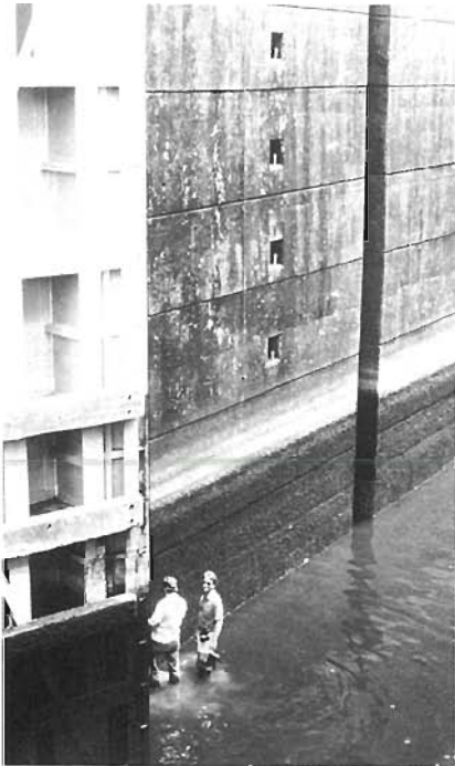
Routine maintenance at the Moss Bluff lock on the Oklawaha River. Spray crews often do more than plant management. Photo by David Girardin.
