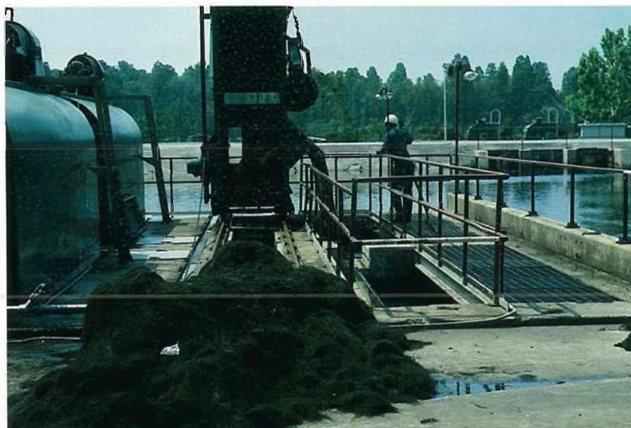
Worker clearing weeds from power plant intake structure during an episode of weed impingement.
